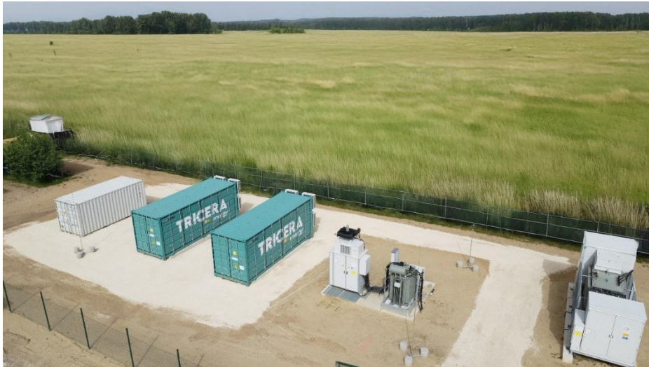
Image: Stock photo of a battery storage system from TRICERA energy
