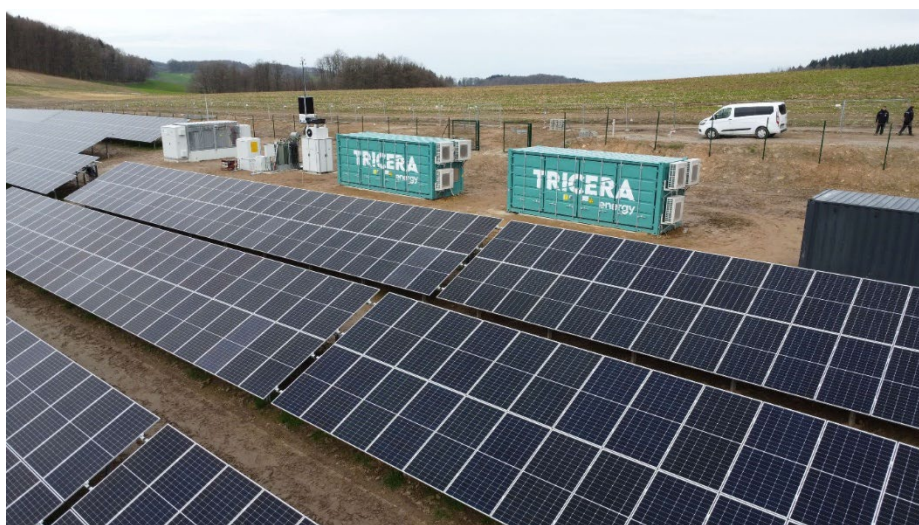
Photo: Aerial view taken with a drone of the battery storage project with ABO Energy in Wald-Michelbach
