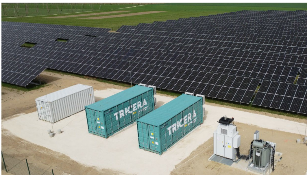
Image: TRICERA energy battery storage system in operation from a project with ABO Energy
